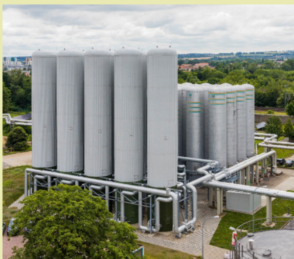
Thermal storage at the Reick Innovation Power Plant, SachsenEnergie, Killig 2021.
