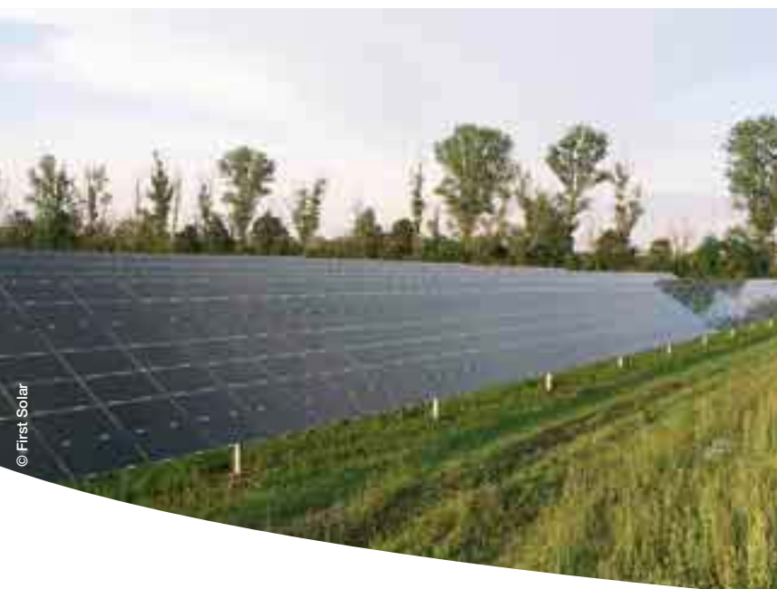
Large PV power plant with thin film solar Modules
