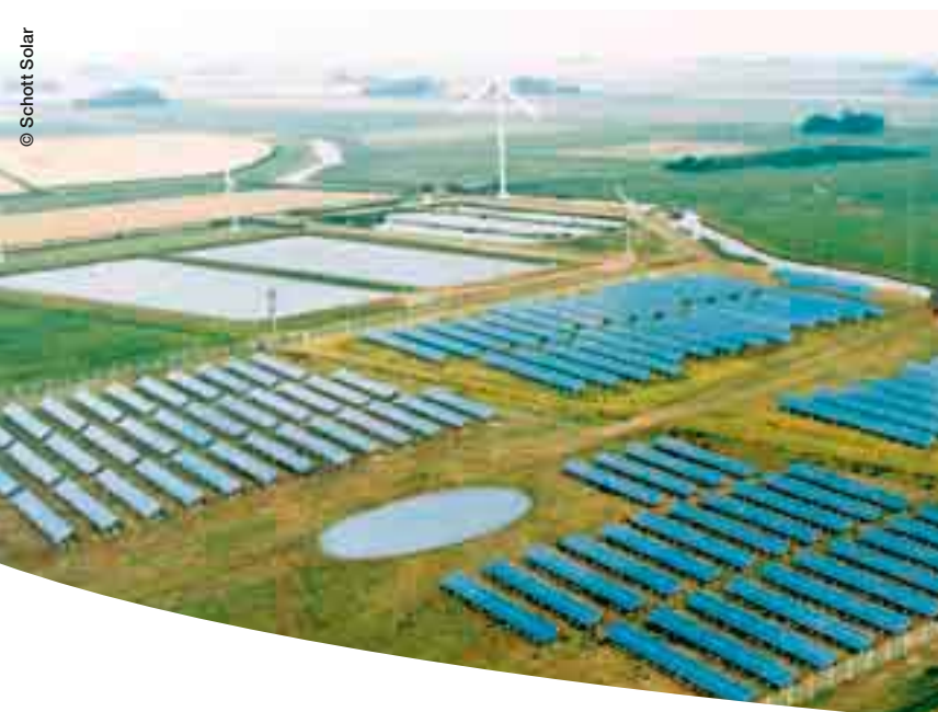
PV plant in Pellworm
