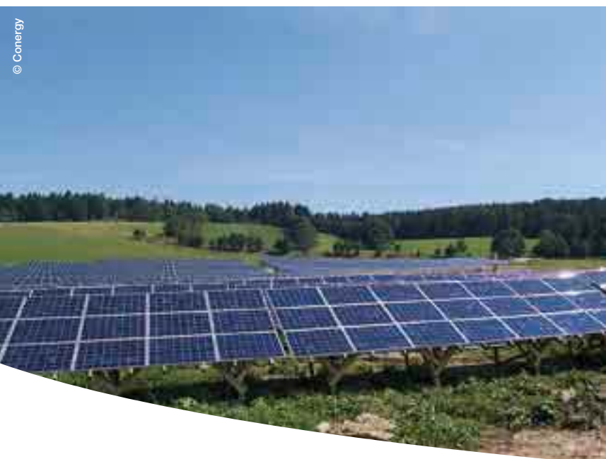
Large PV power plant
